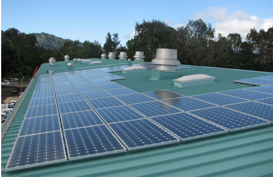
Figure 8: Photovoltaic Panels at the DOT Highways Division Baseyard in Līhu‘e
